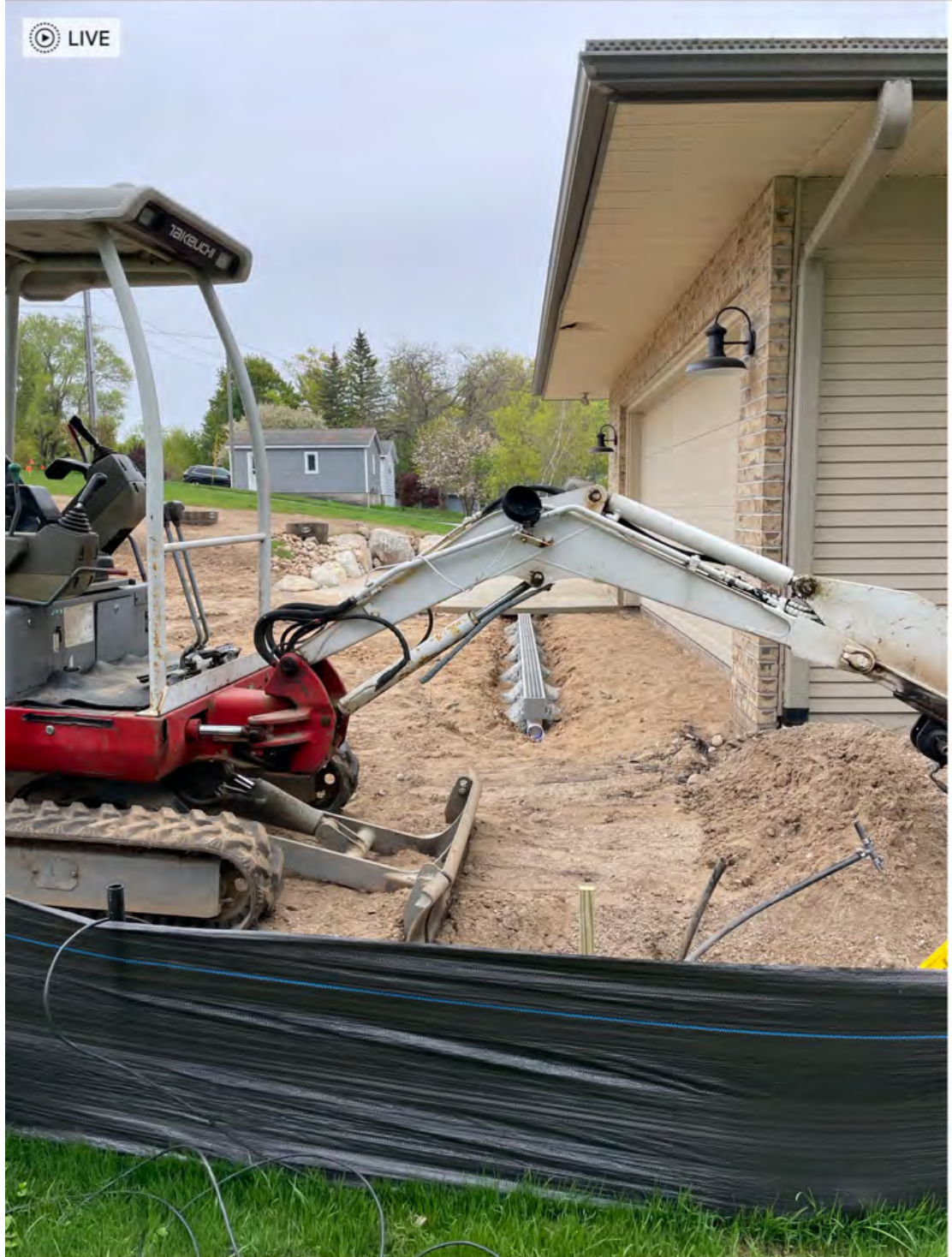
May 14, 2023 New trench drain with output toward 1669 Lake Drive Excavation and fill dirt, Lower concrete completely removed.
