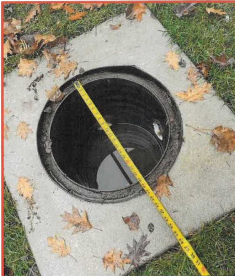
12/23/23 Photo 2 Upstream Catch Basin with no perforations noted and standing water in the sump.
