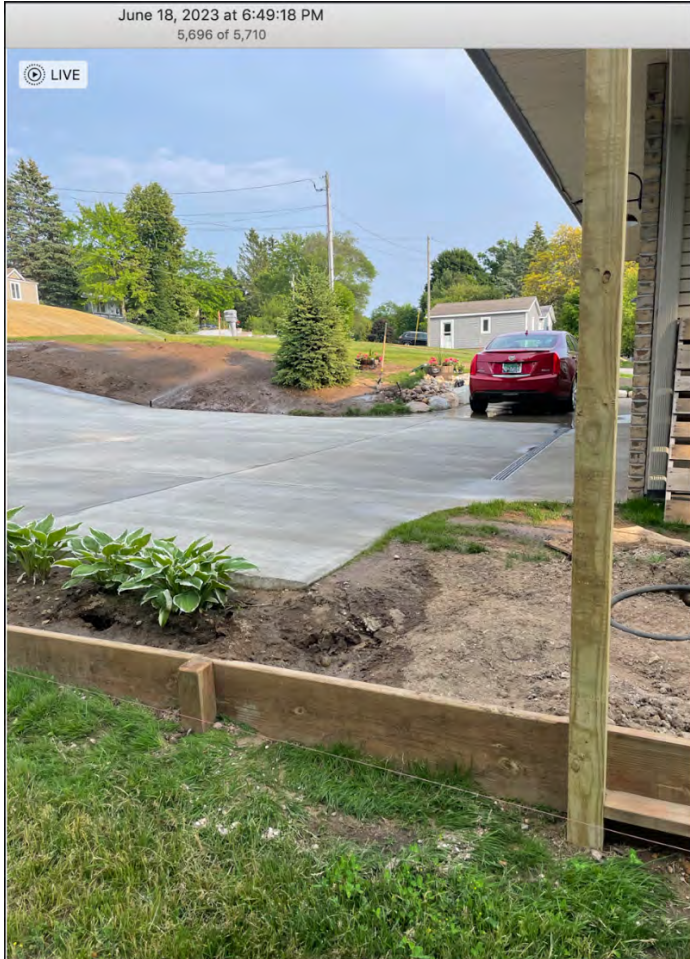
Notice the washout in the foreground from the sprinklers running on the opposite side of the driveway. The riser is buried between the corner of the garage and the 1669 property border. Drainage from the 1661 Driveway routinely overflows the retaining wall at this location. The elevation of the 1661 property has been increased by over 11 inches.
