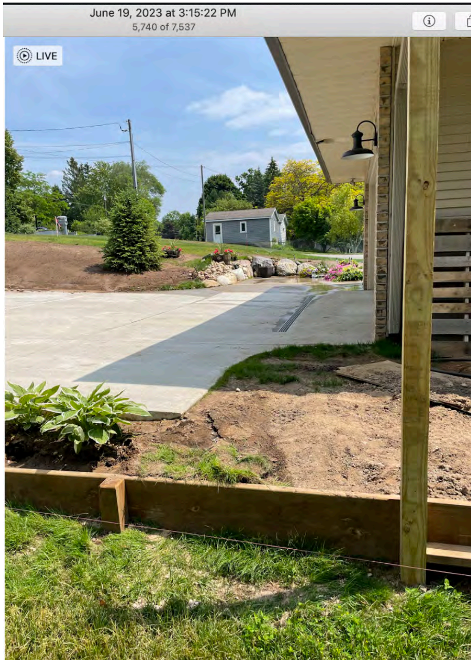
Clear view of the new South parking pad. Notice the running sprinklers on opposite side of the property create drainage at the 1669 property border.
