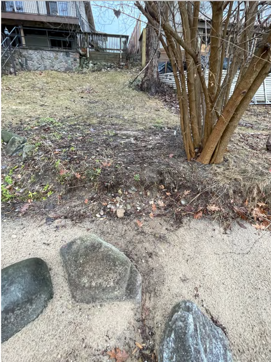
Continued washout at same location after the first Spring storm March 2024
