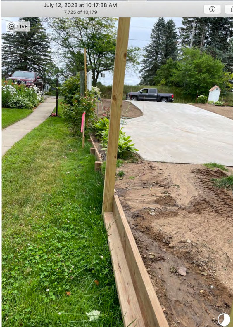
Direct runoff from concrete in 10 foot setback sends water to the retaining wall, where it escapes onto my property
