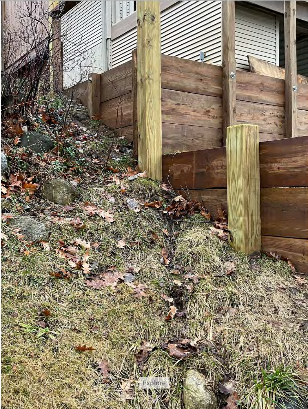
Water path from corner of the Lower drain where water exits at the base of the drain.
